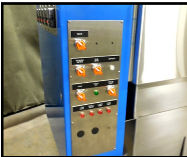
Simple Control Safety Panel
