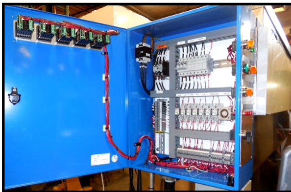
ULTRA — Electrical Panel with sophisticated temperature display & indicator light system
