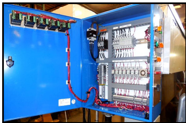
ULTRA Model VS-5 Electrical Panel with sophisticated temperature display & indicator light system
