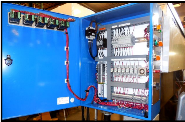
ULTRA Model VS Electrical Panel with sophisticated temperature display & indicator light system
