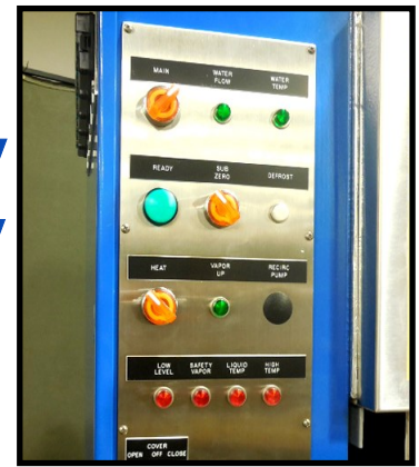
Simple Control Panel with Comprehensive Indicator Lights
