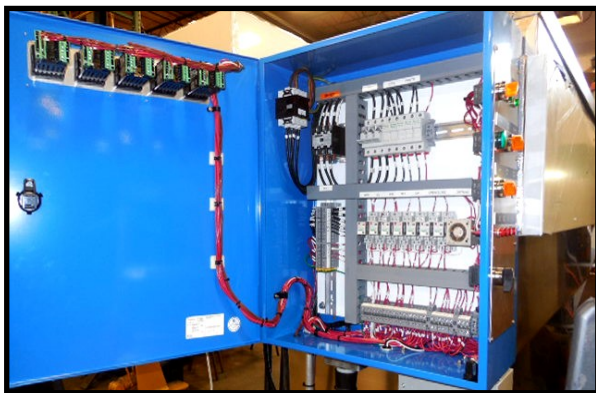
ULTRA Model VS Electrical Panel with sophisticated temperature display & indicator light system
