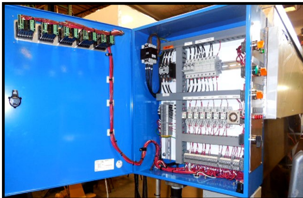
ULTRA VS-4012 LE—Electrical Panel with sophisticated temperature display & indicator light system
