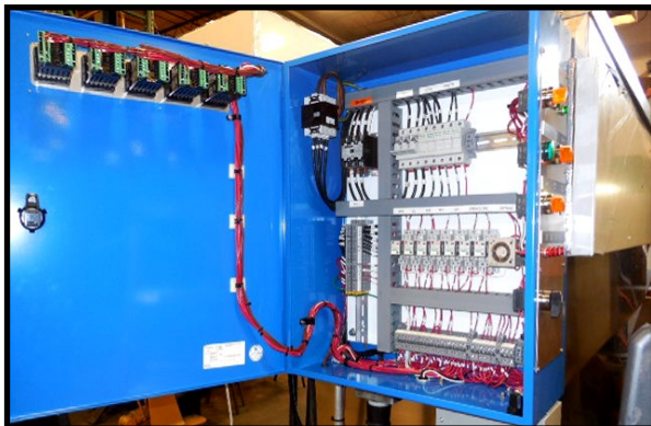
ULTRA VS-2 (2418)LE—Electrical Panel with sophisticated temperature display & indicator light system
