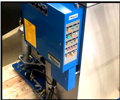
Simple Control Safety Panel
