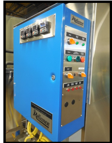
Simple Control Safety Panel
